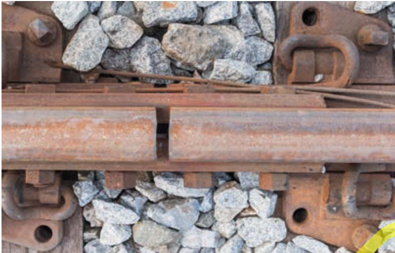
FIGURE 1 Expansion gap left between the old railway lines
