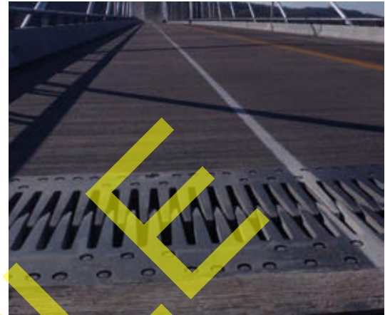
FIGURE 2 Thermal expansion joints, such as these in the Auckland Harbour Bridge in New Zealand, allow bridges to change length without buckling.
